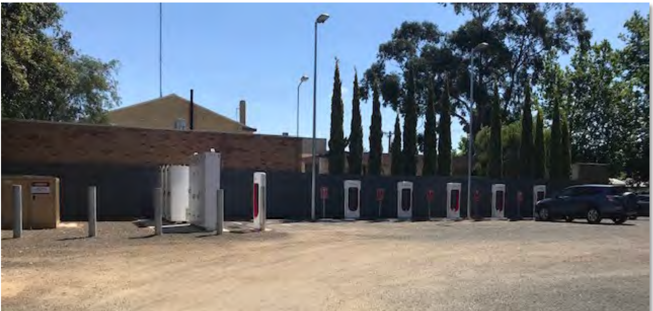
Figure 10: The Tesla Super charger site in Euroa is located in a public off-street car park opposite a public toilet and within walking distance to the main street
