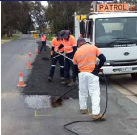
We dry sealed the cracks in the road on Waller Street. This helps prevent water getting under the seal.
